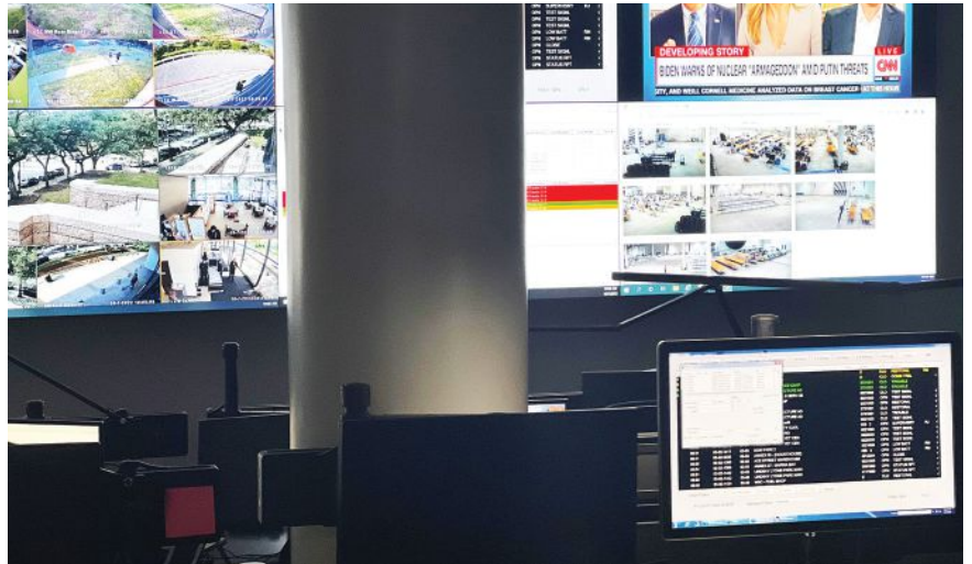
Harris County's Security Technology Services division feeds all IP cameras, access control, body-worn cameras, intrusion detection systems and fire monitoring into its SOC, which includes a 24/7 emergency response call center.
